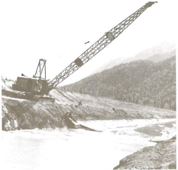
Excavating tailrace channel, 1954. The bottom of the channel is below the ground water table, resulting is seepage into the channel.
