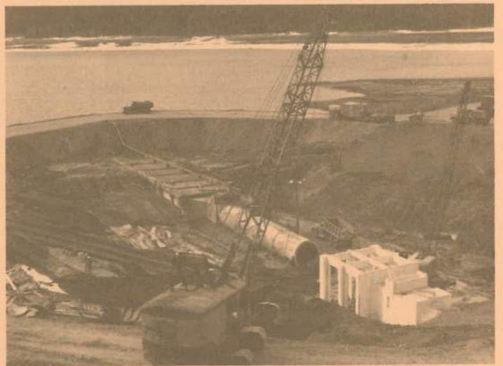
Rebuilding the intake structure, 1965. A temporary coffer dam was built to allow dry access to trashgates, concrete conduit pipe, and bulkhead structure.
