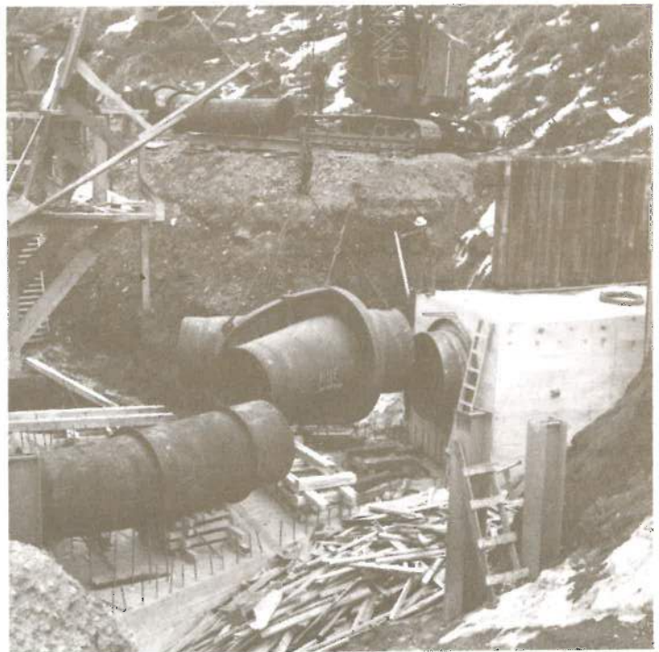
Installing penstock wye at powerplant, 1954. The wye splits water in the penstock into two streams, one stream for each turbine.
