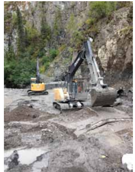
Tundra mats in use to allow machinery to operate on unstable sediments.
