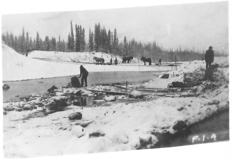
Figure 5 Eklutna Lake storage dam under construction. Nov. 21, 1928. Looking north from lower end of spillway channel toward
